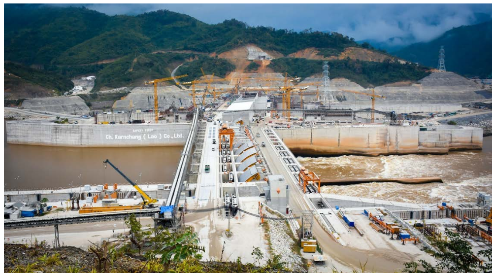
Construction of the Xayaburi dam and hydropower plant on the Mekong River, Laos. Image by Onutto.
